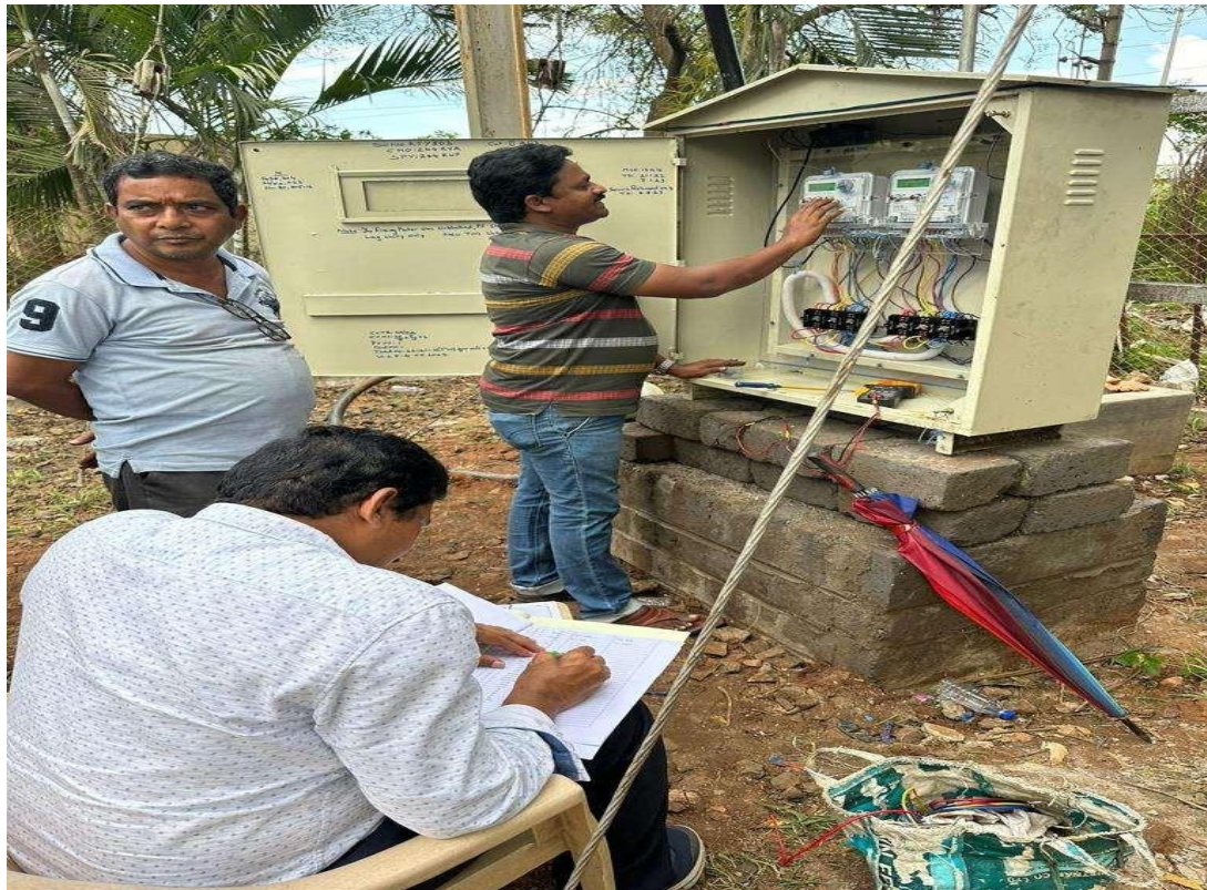
Net metering from APEPDCL @ Power House
