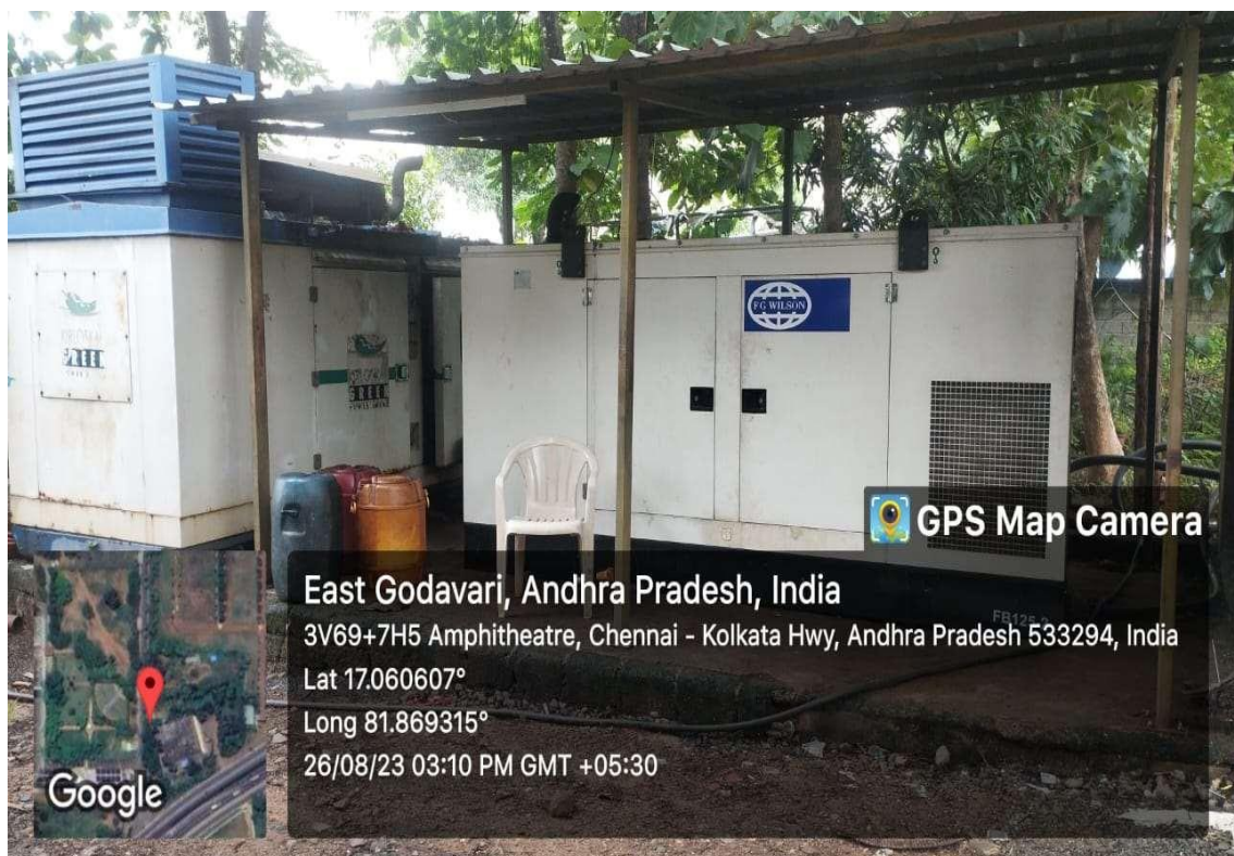
Diesel Generator @ Power House
