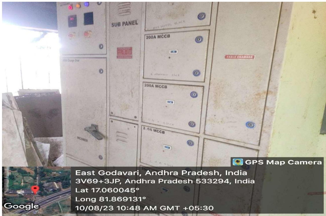
Power Control Panel @ Power House
