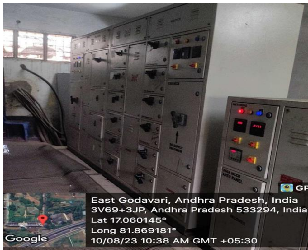
Power Control panel @ Power House
