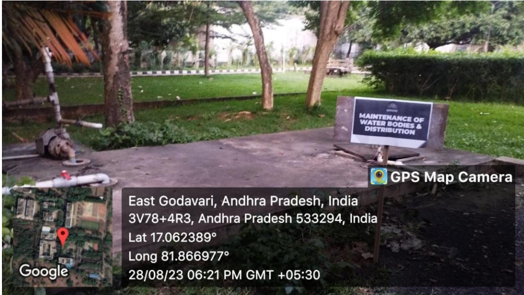
Water stored in Closed Tank for Distribution
